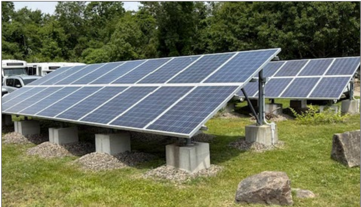
Figure 71. Solar Panels at CATA
